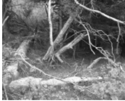
Overgrown foundation of side of main house.
